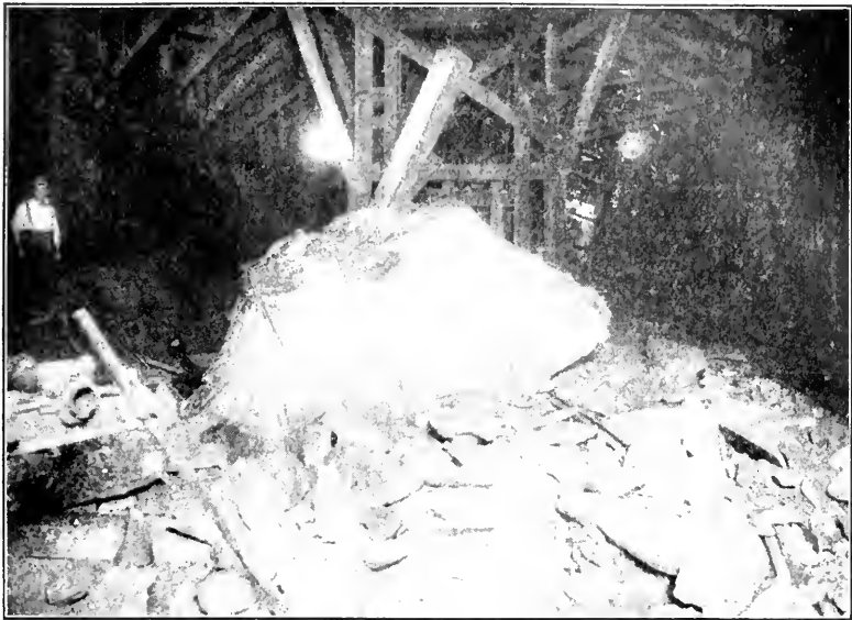
FIG. 7.—BLASTING FOR DEEPER LEVEL: ILLUSTRATING THE FACT THAT, WITH AMPLE CLEARANCE, THERE IS ABSENCE OF DANGER.
